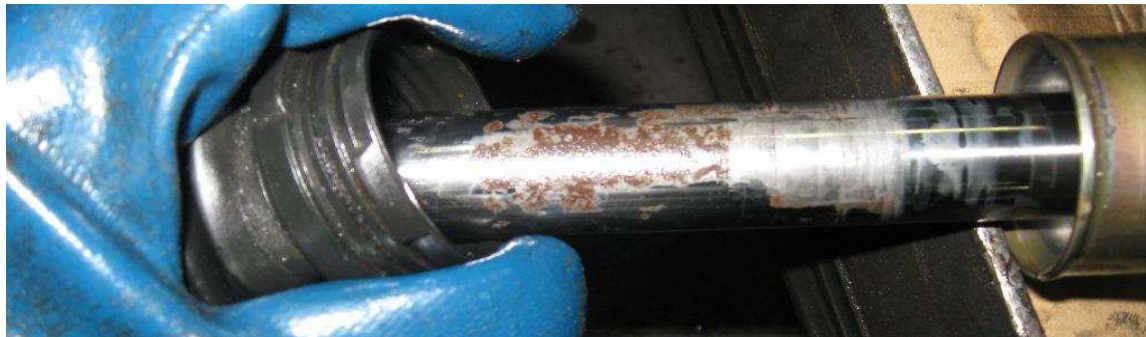
NOT GOOD - Rusty rack
